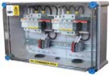
Dual String Combiner box with 1000V DC Isolator, Surge protection, String Fuses, Terminal connectors for input and output
