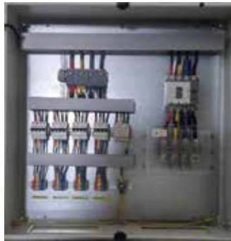
Three Phase Distribution box for combining four Inverters, includes Circuit breakers for each inverter, Molded case circuit breaker and Surge protection in output side.
