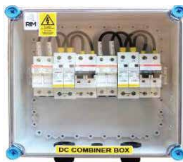
Three Phase Panel DB for Load Sharing with Solar Dual String Combiner box with Circuit breaker, Surge protection and String Fuses for each string
