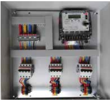
Three Phase Panel DB for Load Sharing with Solar meter, Circuit breakers for Solar Side, Grid Side and for Load side
