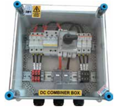
String Combiner box with Three inputs with fuses on each string and Three outputs with one isolator and one surge protection device.
