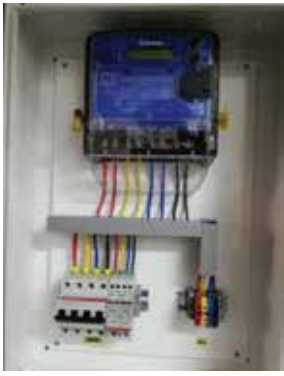
Three Phase Combiner box with Solar Production meter, Surge protection device and Circuit Breakers
