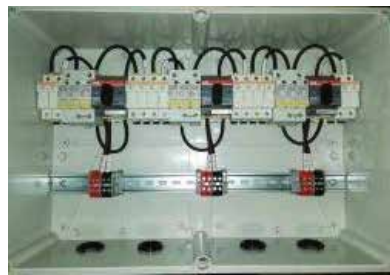
String Combiner box with Six inputs with String fuses and Six outputs with three isolators and three surge protection devices
