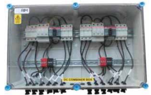
String Combiner box with Six inputs with String fuses and Six outputs with two isolators and two surge protection devices, output connections through panel connectors
