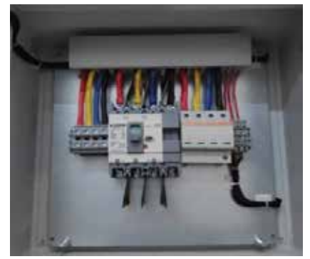
Three Phase AC Combiner box with Surge protection device, Molded Case Circuit Breaker with rating of 100A and RYB indication
